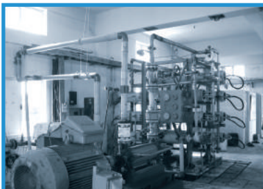
Supply and Installation of Multistage Pump- 61.0 Bar for Desalination Plant
