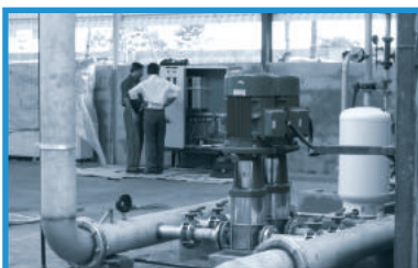
Supply and Installation of Pressure Feed Pumping System for Soft Flow Deying Unit
