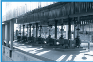
Supply and installation of Pressure feed pumping system
