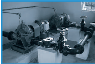
Supply and Installation of HSC Pumpset for Water Supply Project
